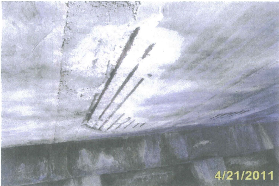
Photo #3 Element 39 - Delamination in underside of Slab Unit 1-5 at the 1/4 point
