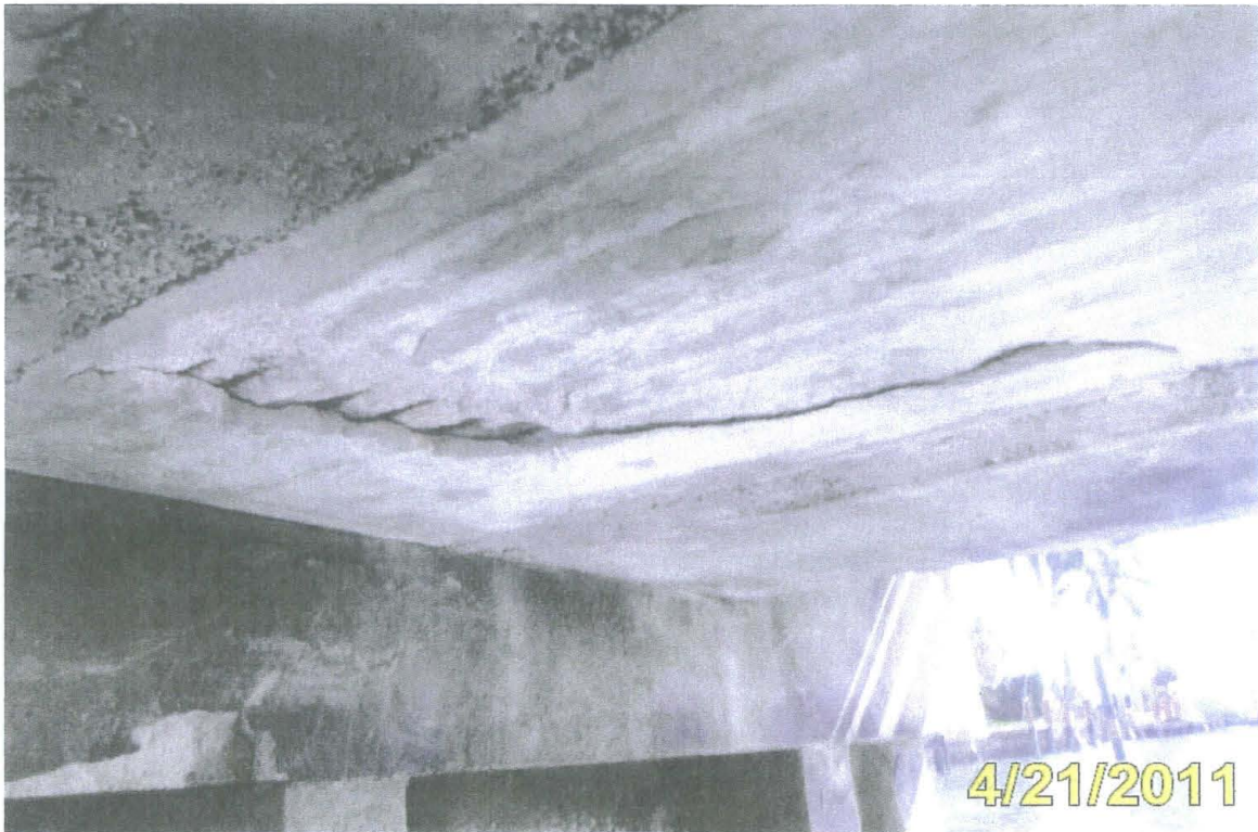
Photo #4 Element 39 - Delamination and spall with exposed rebar in underside of Slab Unit 1-5 at 3/4 point
