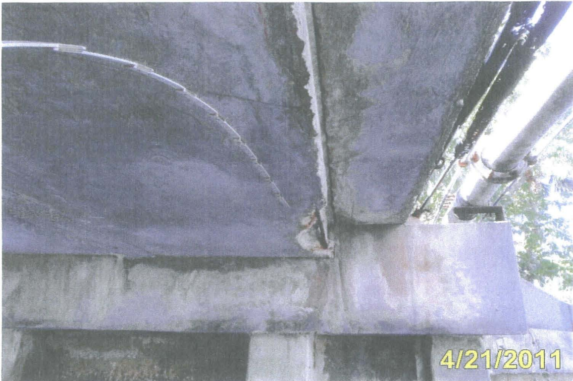
Photo #1 Element 39 - Spall with exposed rebar in west edge of Slab Unit 1-1 at Abutment 1
