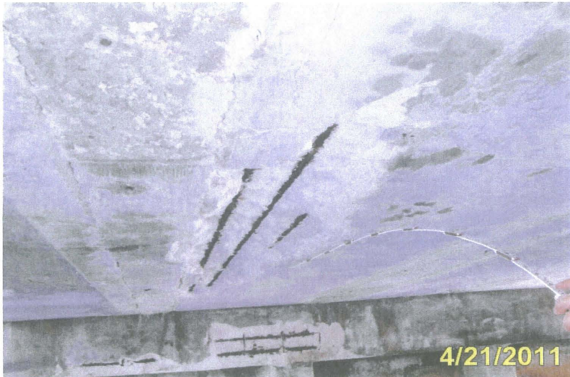
Photo #2 Element 39 - Delaminations and spalls with exposed rebar in underside of Slab Unit 1-2
